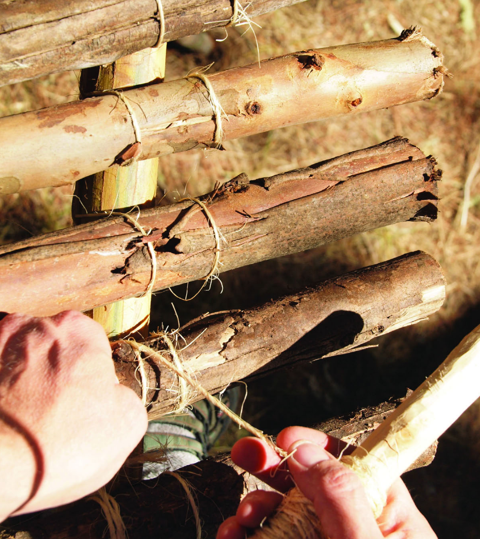
Figure 8-19 You can run the lashing between many sticks at once to create a quick decking.
