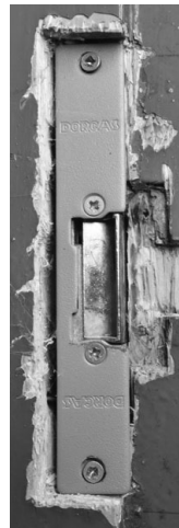
FIGURE 6-2: THE ELECTROMECHANICAL DOOR LATCH
